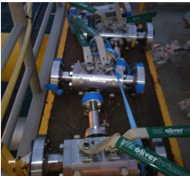
Methanol System PCV Valves
