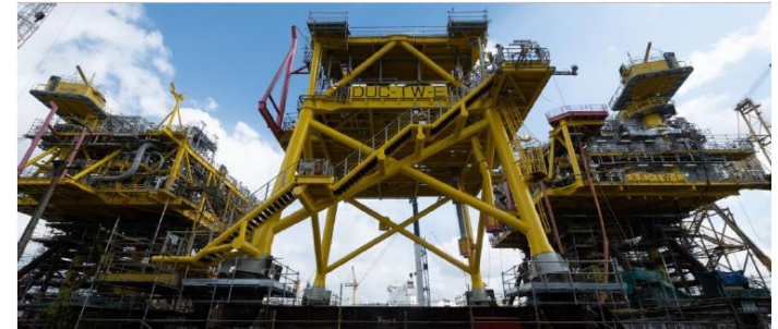
The final look of the Tyra West facilities at the SMOP yard in Singapore before load-out
