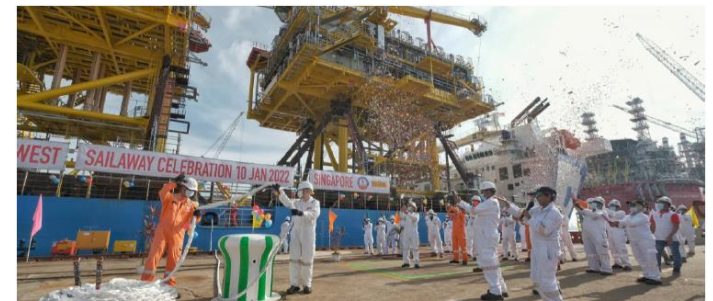
On 10 January at 9:48AM (local time), the Tyra West facilities and two bridges were sent off
